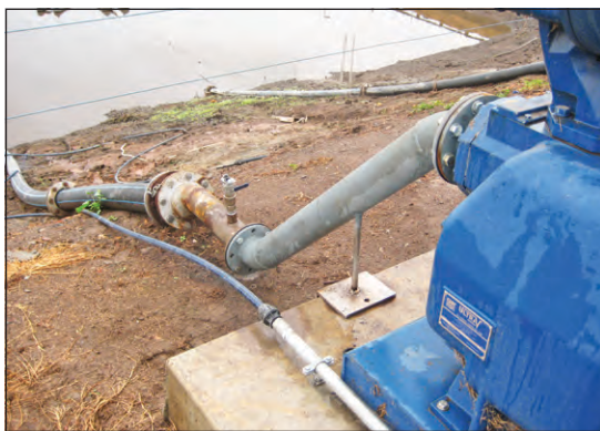
The Gorman-Rupp VS3A60-B pump has operated with minimal operator intervention for the past six years.
