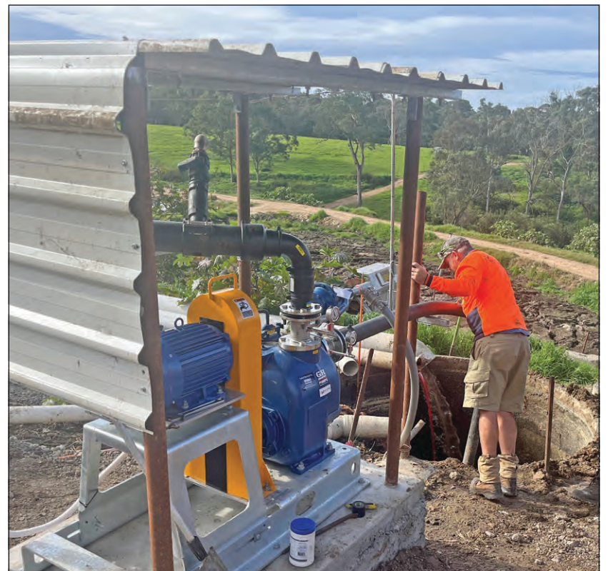
Within a day of operation, the Gorman Rupp Super T3C60SC-B, fitted with the solids management system, had waste material pumping steadily to the separator screen.
