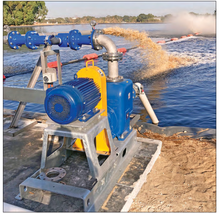
The EchoStorm venturi aerator was the solution, supplied by Hydro Innovations.
