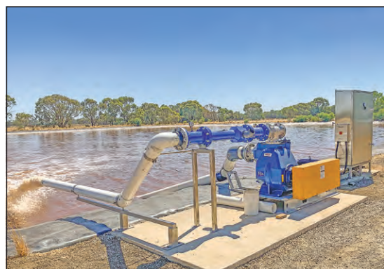
The lagoon two weeks after the installation of the Venturi Aerator. Ripples from the aerator that radiate to all parts of the lagoon ensure a good level of mixing.
