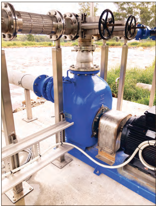
Gorman-Rupp 'Super T Series' self-priming wastewater pumps are easily accessible for monitoring and maintenance.
